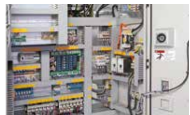
C. Electrical box Neat and clear wiring configuration
